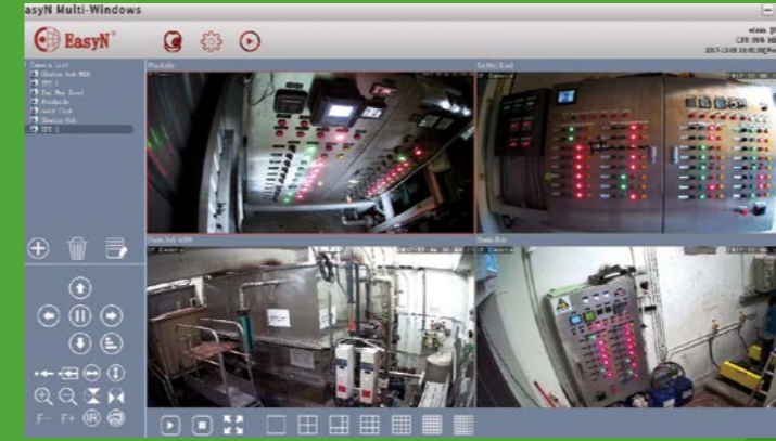
Real-time camera monitoring system
